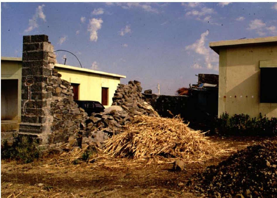
Figure 10: A newly built stone wall at new Sirsal village that collapsed in 1996 after only 2 monsoon seasons. Photo courtesy of Rajendra Desai.
