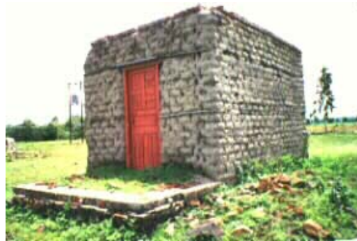
Figure: Model House to demonstrate earthquake safe construction lying in ruins.
