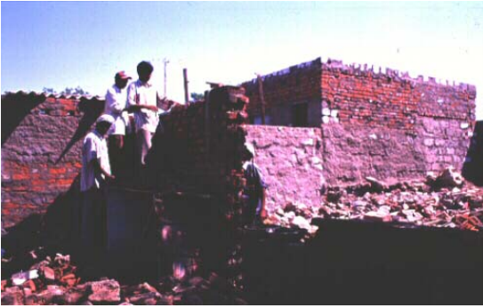
Figure Above: Poor self-help construction using combination of materials in Bhachao
