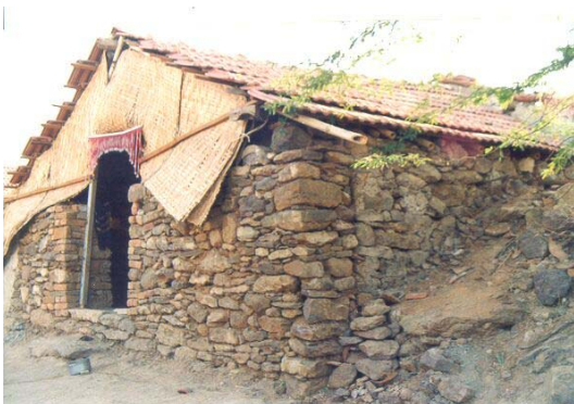
Figure: Semi permanent shelters are already getting permanent by raising walls in stone, without consideration to earthquake safety
