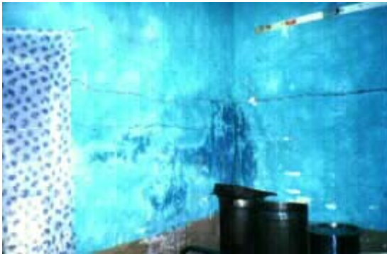
Figure: Cracks in the newly reconstructed villages from a mild earthquake.
