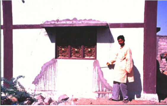
Figure: Wrong repairs by filling through cracks with cement grout in Village Nani Cherai.
